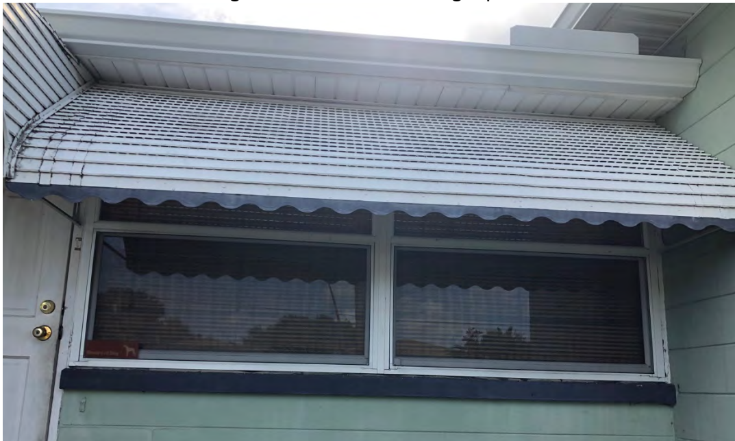
Image 12: Windows not being replaced
